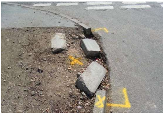
Loose or missing kerbs
