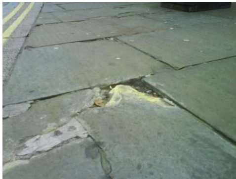
Level difference to broken/damaged flags
