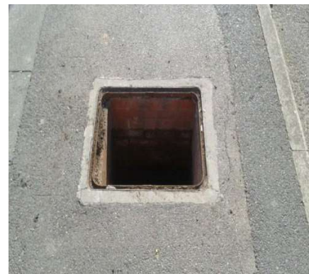
Missing Manhole Cover
