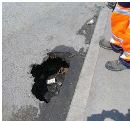
Collapse in Carriageway
